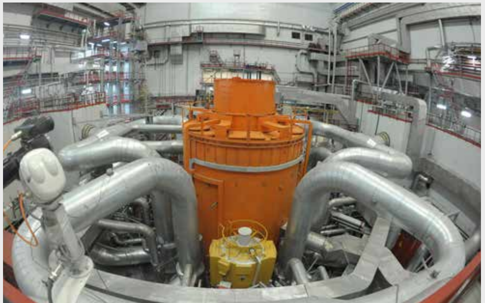
The reactor vessel and coolant piping of the BN-800 in Russia, one of the few operating sodium-cooled fast reactors in the world. UCS found that these reactors can pose unique safety issues, as their sodium coolant can burn when exposed to air or water.
