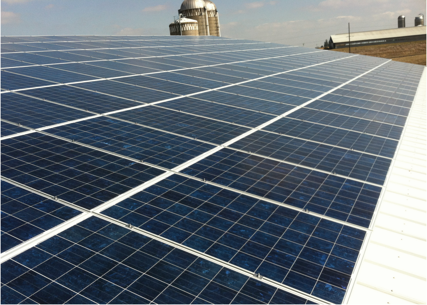
In 2012, Gibbs Dairy, in southeastern Minnesota, installed 166 solar panels that are expected to supply the farm with 30 percent of its electricity needs annually.
